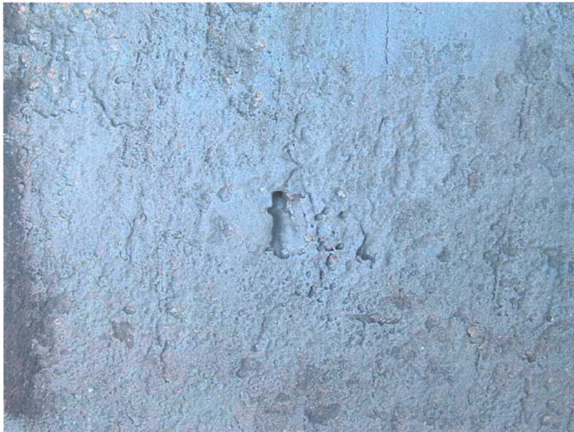
Image 20 – Deep Corrosion Pitting
