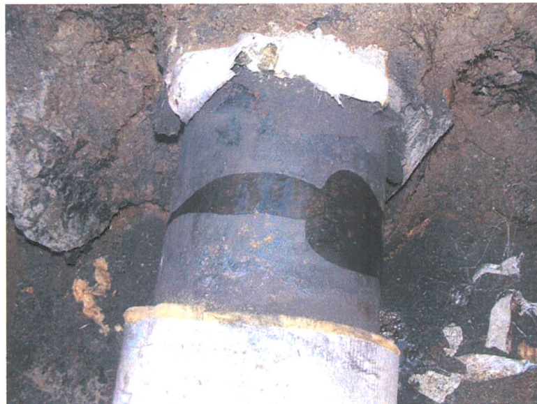
Image 21 – Exposed Water Main within Trestle
