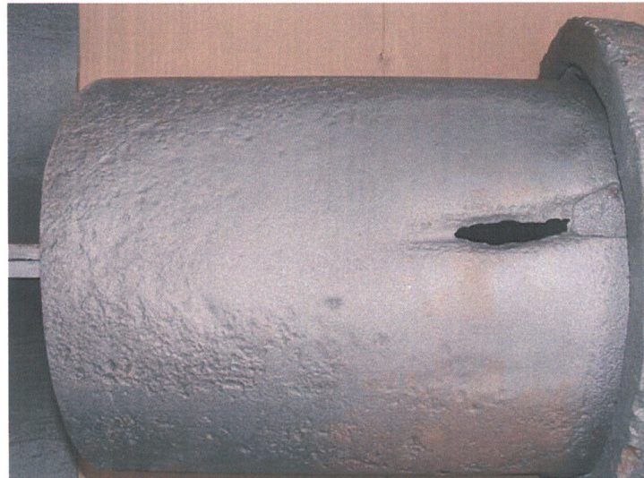
Image 33 – Erosion Hole from Exterior
