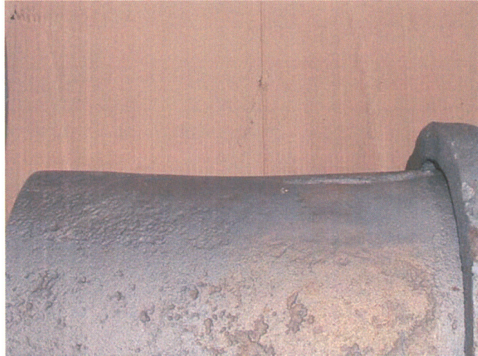
Image 35– Erosion under Repair Clamp
