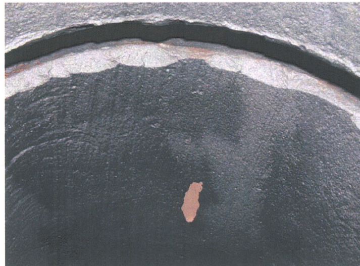
Image 34 – Erosion Hole from Interior
